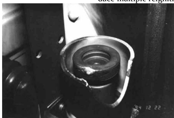
Fig. 1 Damaged vacuum breaker tube
